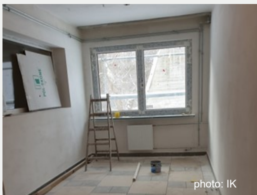
Photo 5. General view of a new laboratory room in Building 26 where absorbers for EMC chamber will be stored
