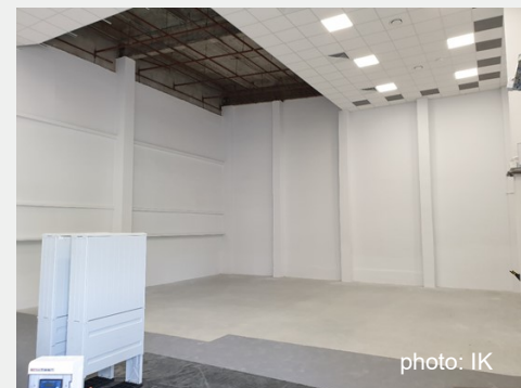
Photo 8. View of the hall in Building 26 where SAC-3m EMC semianechoic chamber will be constructed; stage 2
