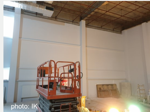
Photo 6. View of the hall in Building 26 where SAC-3m EMC semianechoic chamber will be constructed; stage 1
