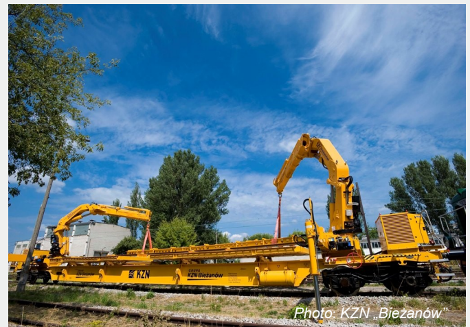
Fig. 3. Loading and unloading of the railway turnout from the vehicle with HDS cranes
