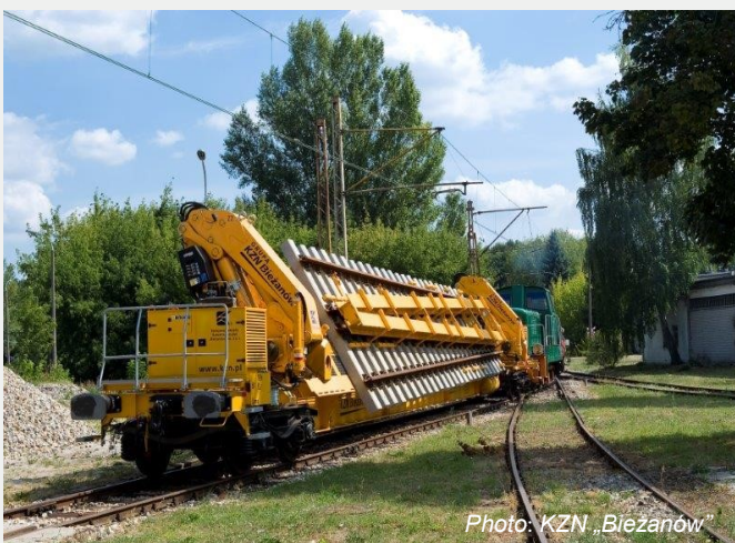
Fig. 4. KZN01A type vehicle loaded with a railway turnout. The turnout is additionally stiffened by a dedicated protection system
