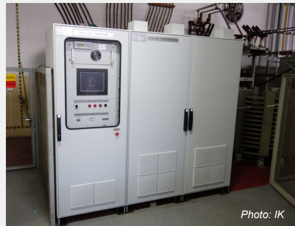
Fig. 2. Energy storage DC/DC converter
